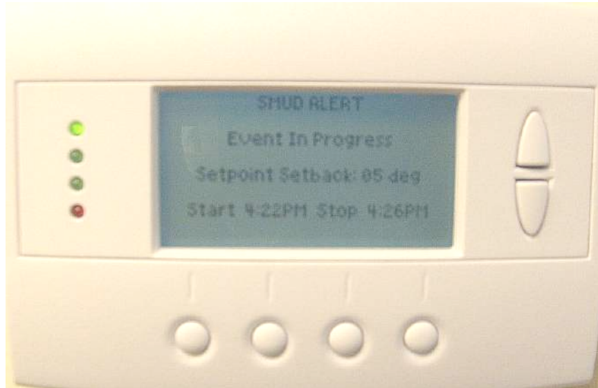
Figure 68. Programmable Communicating Thermostat Displaying Ttemperature Event in Progress Notice
