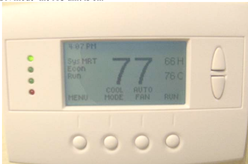
Figure 61. Programmable Communicating Thermostat Showing Current Settings Before Tier 4 Event
