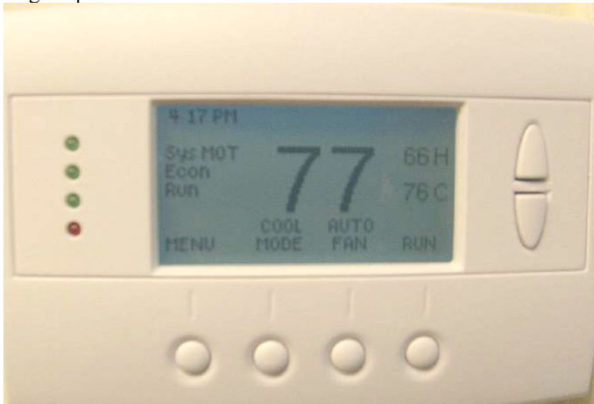
Figure 67. Programmable Communicating Thermostat Displaying Current Settings Before Temperature Event
